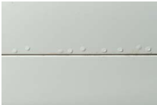
Condensation on the ceiling. Prevent condensation from dripping on meat or work surfaces and thus contaminating the meat.
