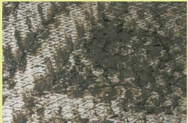
When forklifts drive in and out storage rooms and trucks, they spread dirt all over. Make sure floors are clean to start with.
